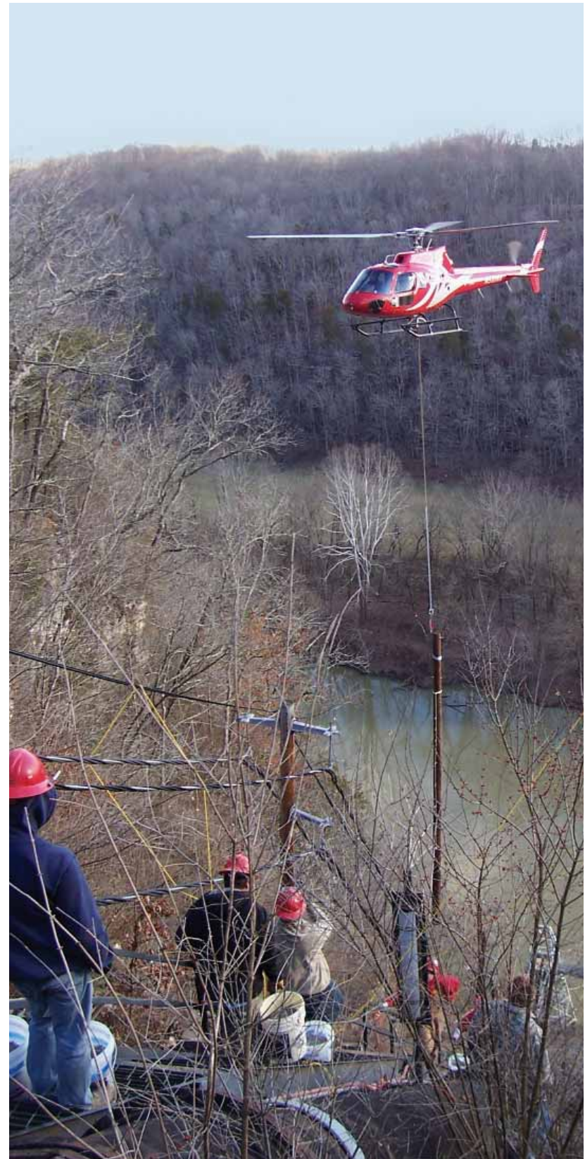
St. Louis Helicopter transported and placed a power pole during the recent electrical power supply upgrade made to Nicholasville's raw water intake at the Kentucky River.
